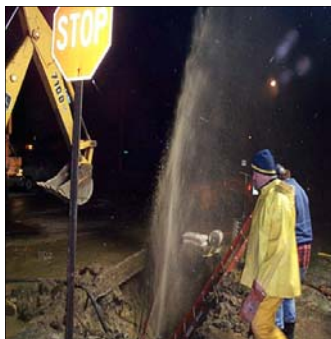
DPW attends to a Water Main Break.
